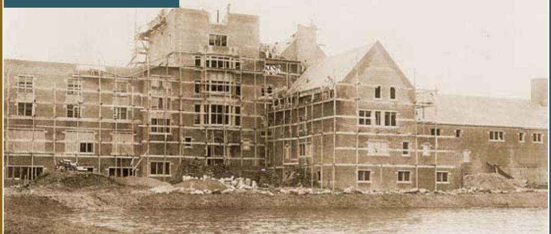
Horace Dutton Taft Hall, designed by renowned architect Bertram Goodhue, under construction in 1912–13, proved to be a seminal space, and every building on campus since has carried on an architectural dialogue with it. Note the kitchen wing on the right and the view from Headmaster's Circle, inset. LESLIE D. MANNING ARCHIVES
